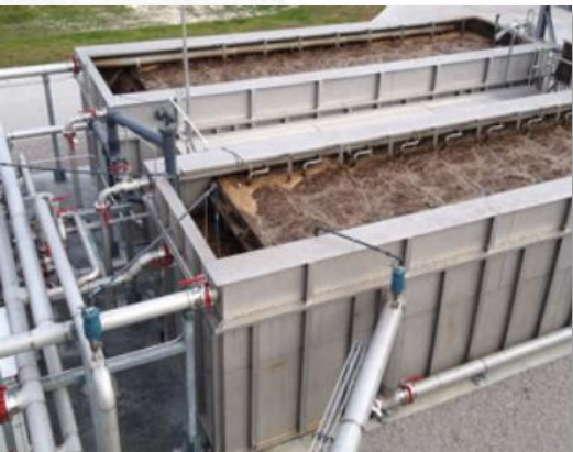
MEMBRANES BIOREACTOR (MBR)
