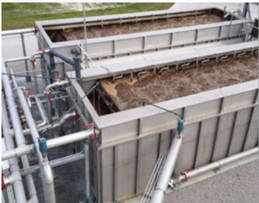
MEMBRANES BIOREACTOR (MBR)
